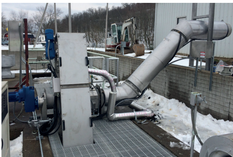
Rittman WWTP 3.0mm micro bar screen catches everything from rags to random bi-products, and is then compacted into pellets and goes into a hopper/compressor.
