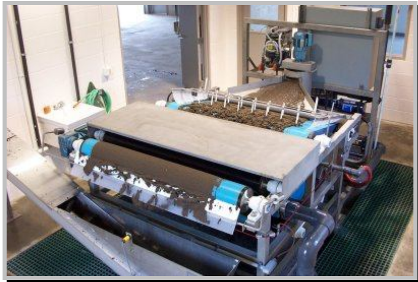
OR-TEC Belt Press System dewatering WAS to 17% solids
