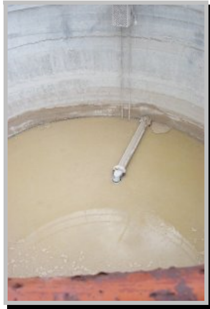
Digester at WWTP with WAS and Lime sludges at 50:50 ratio
