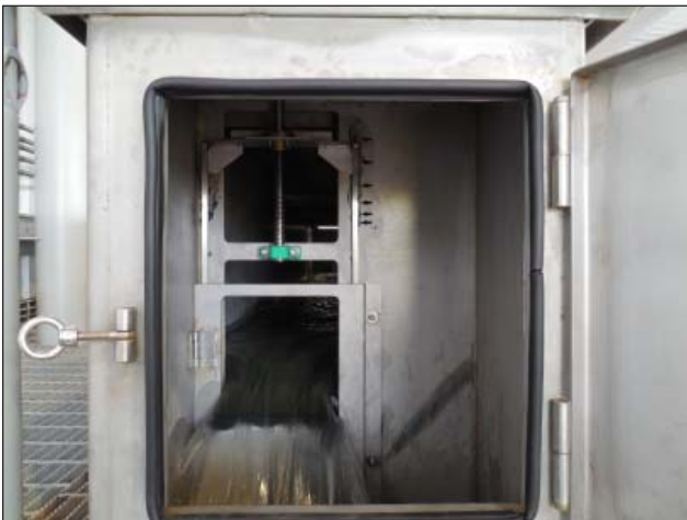
The flow adjusting weir in operation
