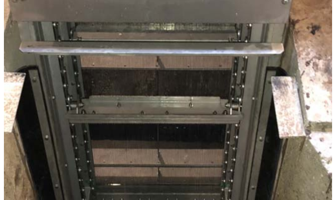
3mm Or-Tec Blue Whale Microbar Screen in Louisville, Ohio wastewater treatment plant.
